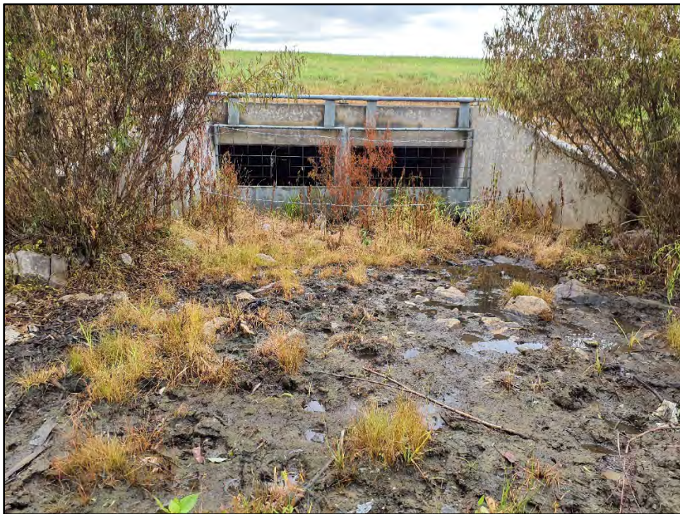
Figure A16. Representative photo of ephemeral stream SA006 within the project area, facing upstream.
