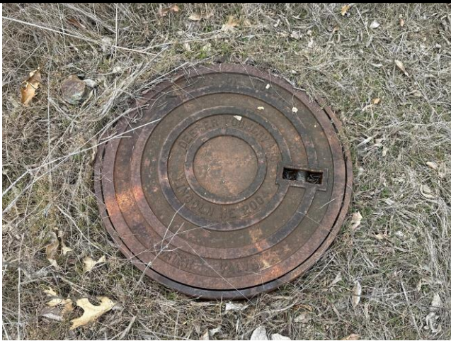
A water valve located in the northwest corner of the Subject Property.
