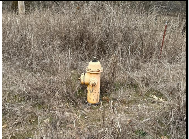
A fire hydrant located in the northwest corner of the Subject Property.
