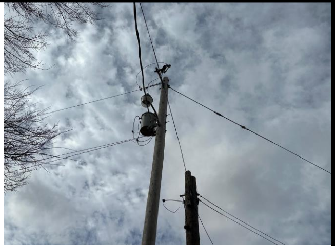
A pole-mounted transformer located west of the residence.
