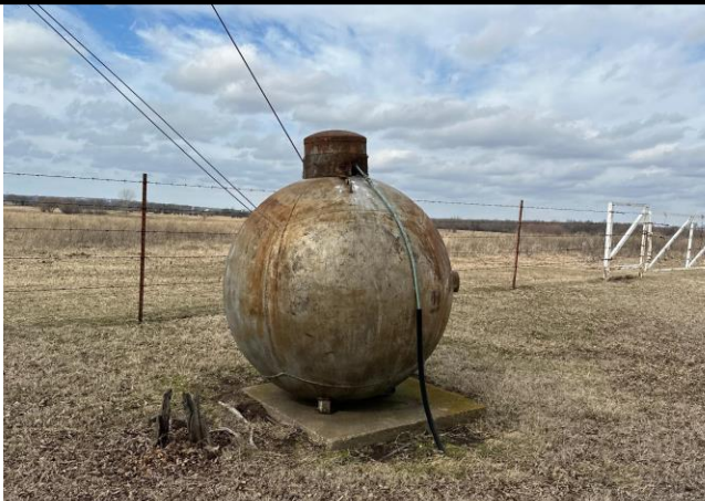
A propane AST located southwest of the residence.
