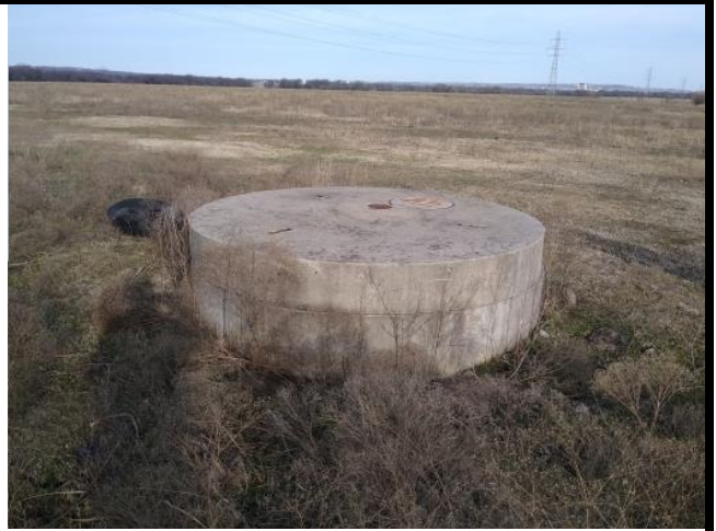
Sanitary sewer system located near the southwest corner of the Subject Property.
