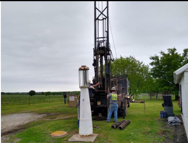
A typical view of the auger rig, with the fuel dispenser visible in the foreground.
