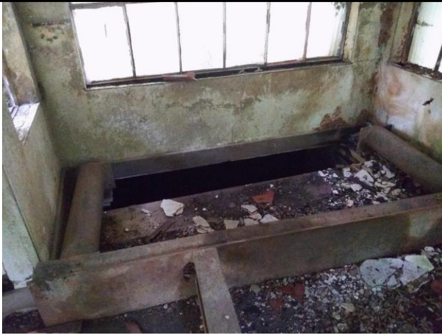
A pit containing liquid inside the scale house.
